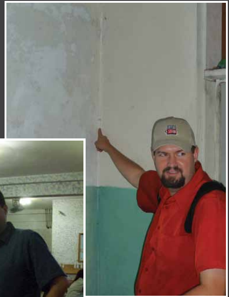
Post-earthquake evaluation of medical clinic building. Very minor cracking at wall corners.
