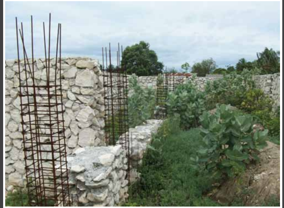
Existing stone masonry walls and concrete column cages to be incorporated into new foundation design for church and school buildings.
